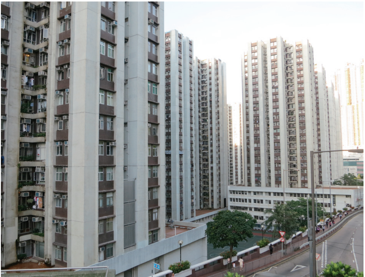
Figure 66: The maintenance of the outside of these residential tower blocks is difficult due to the complex relation between developer, management, and sub-lessees, 2012 (Source: Jesse Rosenstock)
