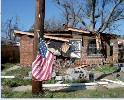
Damages from Hurricane Katrina, © Munich Re
